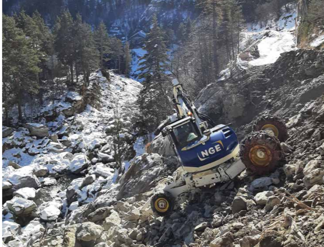
NGE at the bedside of the Roya Valley. Here, the spider excavator carries out the first surveys
