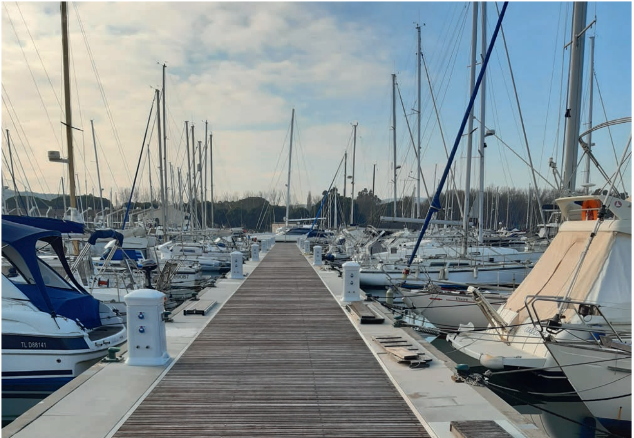
► NGE will connect nearly 500 power and water distribution points in the Port Cogolin Marina
