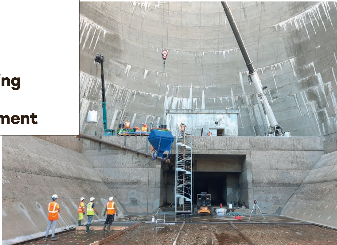
Using UHPFC (Ultra High Performance Fibre Concrete) to upgrade the Soulages holding tank in Saint-Chamond
