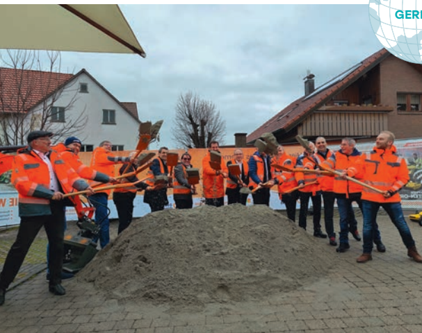
Work begins on the first German fibre connectivity contract in Abstatt (Baden-Württemberg)
