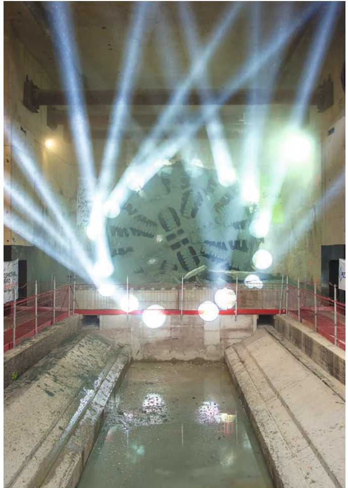
The Sofia tunnel boring machine reaches the end of the line at Serge Gainsbourg station on Line 11
