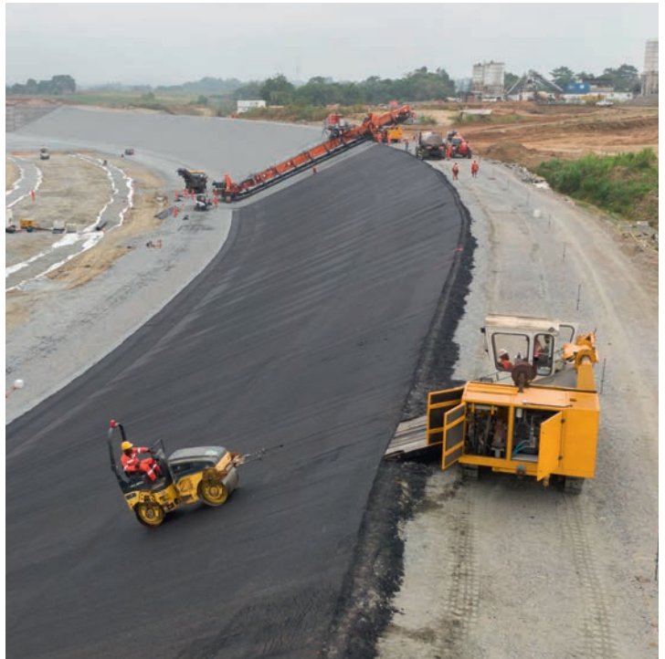
The 35-metre beam paver applies waterproof surfacing to the Nachtigal Dam power channel
